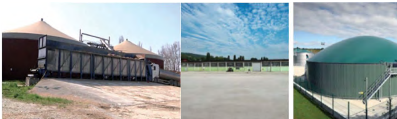
Figure 5. Iraci Borgia biogas plant.
