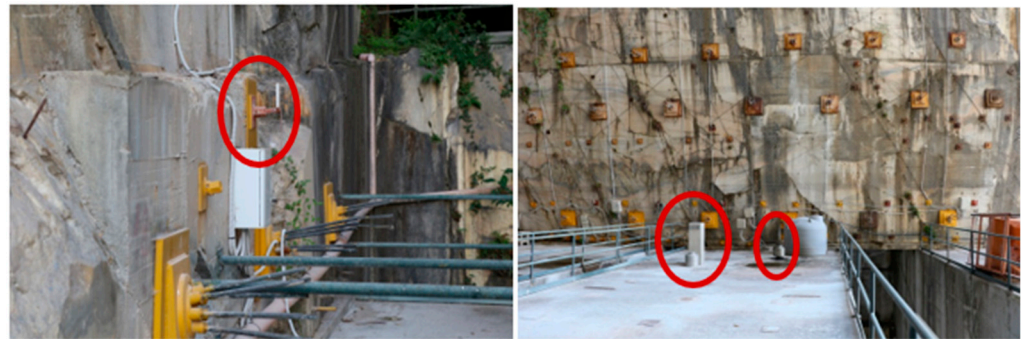
Figure 5. On the left, detail of graduated sights for topographic leveling and wiring for connecting sensors; topographic target inside red oval. On the right, view of the cavern wall with tendons and the suspension terminals of the direct pendulums; measuring points inside red ovals.
