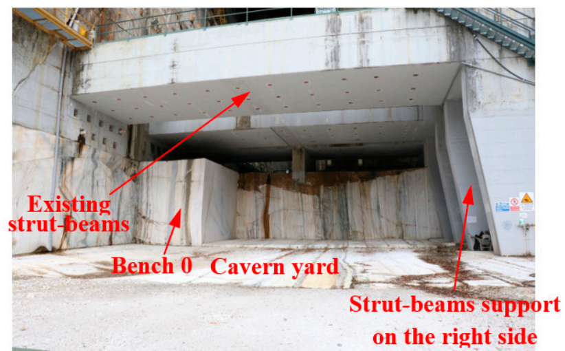
Figure 2. Detail of the first exploitation cut below the beam-struts where the marble extraction works are currently concentrated in the entrance zone of the cavern (Cava Madre of Candoglia).
