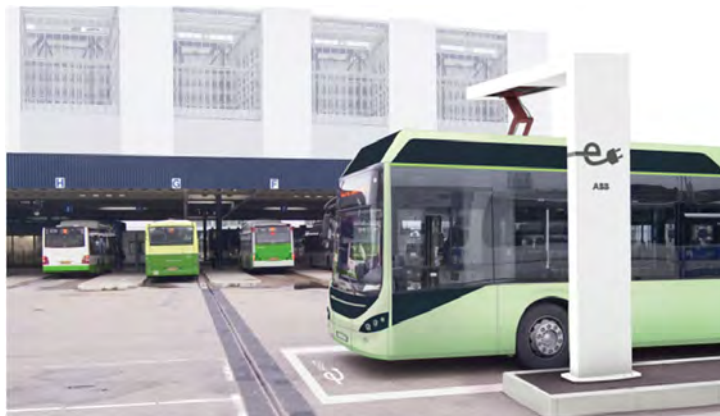
Figure 12. Volvo-ABB charging station.
