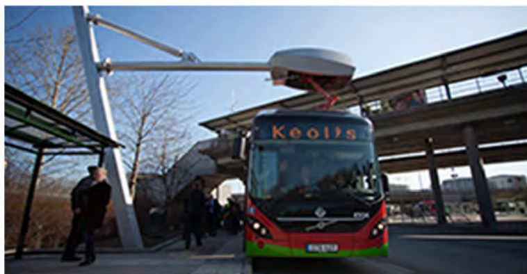
Figure 13. Siemens-Keools top-down pantograph at the charging station.
