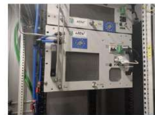
Figure 2 Installed electrolyser at ZEM module
