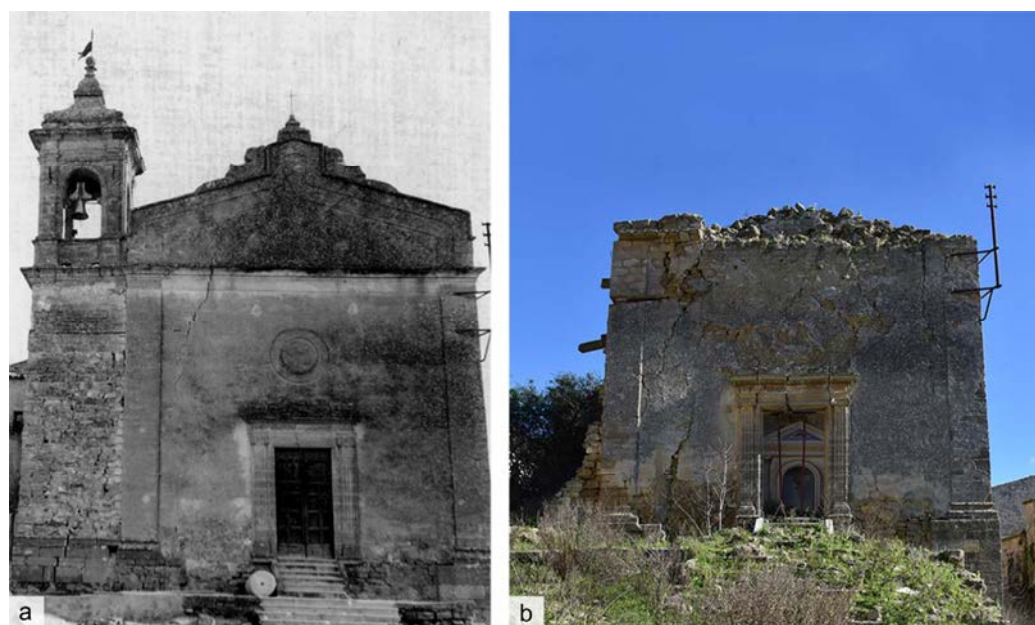
Figure 8. Gesù e Maria Church in the aftermath of the earthquake (a) (courtesy of G. Cocco) and in 2022 (b) (authors' photo).
