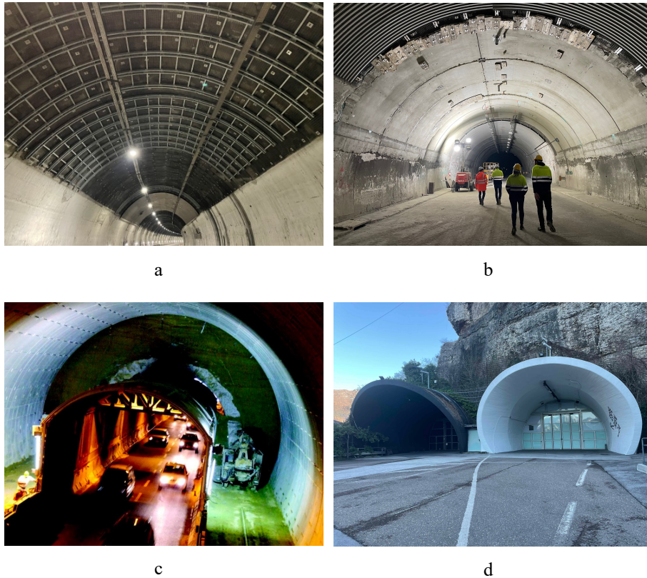
Fig. 1. Examples of strategies throughout coping with tunnel ageing in Italy: a) Provenzale tunnel, Genoa, b) San Fermo tunnel, Como, c) Nazzano tunnel, Rome [2] and d) “Le Gallerie”, Trento.
