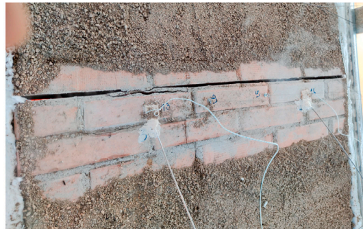
Fig. 10. Failure of brick/mortar interface at arch-crown of vault #1 during the fire exposure.
