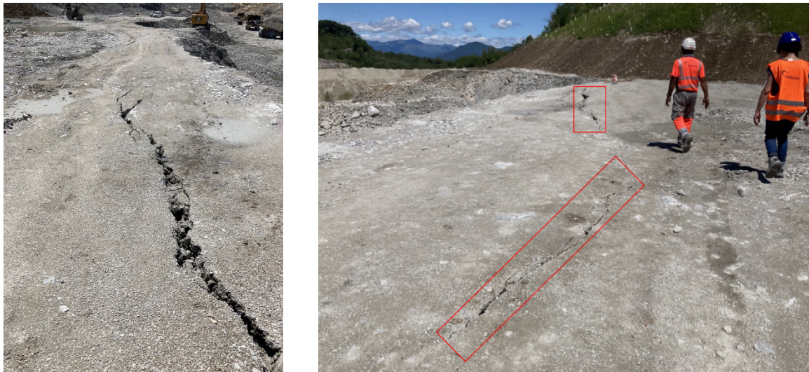
Figure 2. Example of tension cracks formed at the edge of the bench after blasting.
