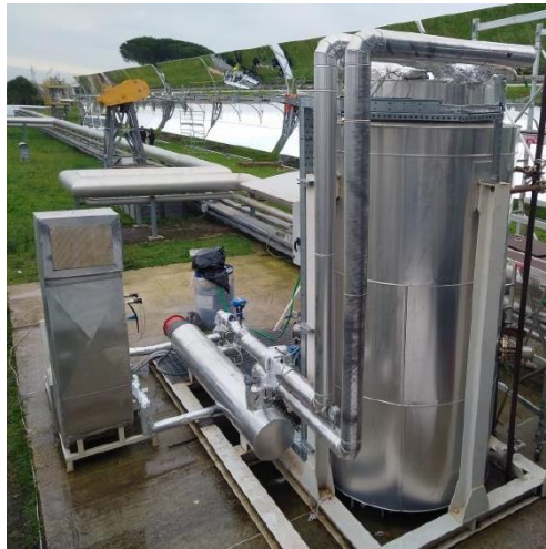
Figure 1. The prototype of the thermocline storage system proposed by ENEA and installed at the PCS facility of ENEA Casaccia (Gaggioli et al., 2020)
