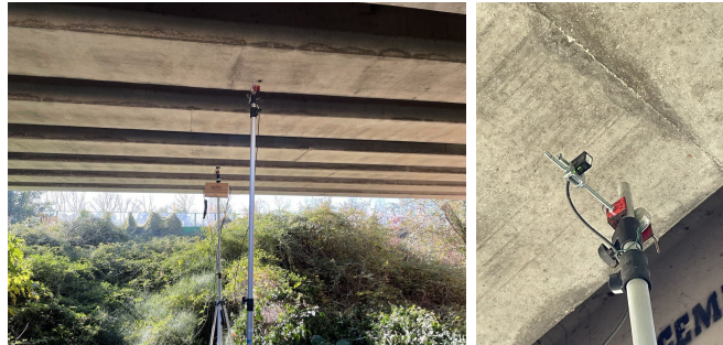
Figure 12: View of the sensors layout and experimental setup in the Orte-Falconara bridge (1st case study) for the bridge deflection measurement using laser sensors under the train transit.
