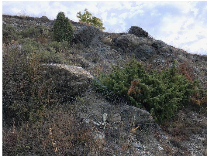
Figure 1. Reinforced drapery system on a rock slope in Sarre, Autonomous Region of Valle d’Aosta, Italy.
