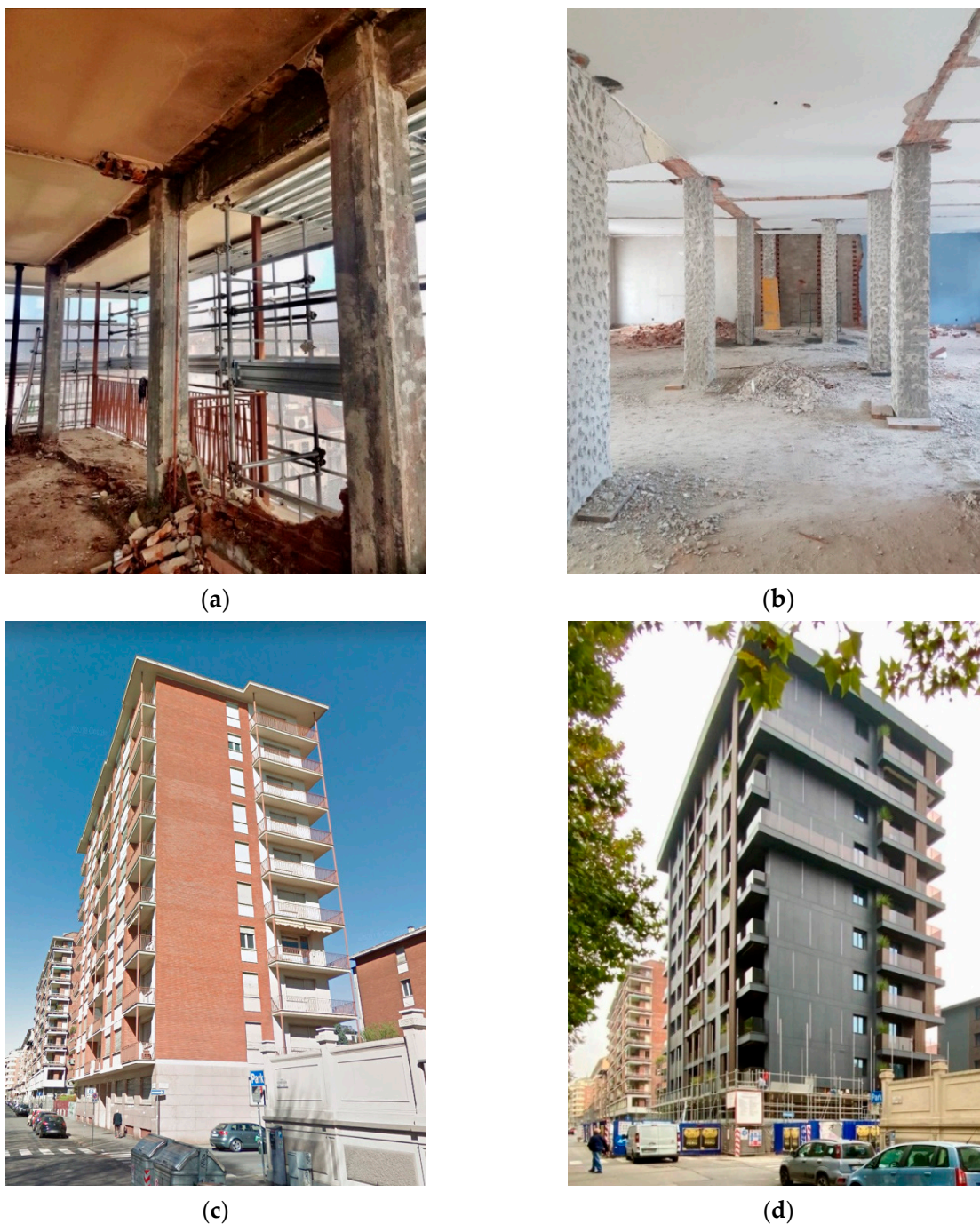
Figure 4. “The Black One”, images of the building site. (a) First phase of the building envelope’s substitution; (b) preliminary phase of the anti-seismic structural reinforcement; (c) the building before the retrofit intervention; (d) the building after the retrofit intervention (photo a, b by Lonero G.) [28].
