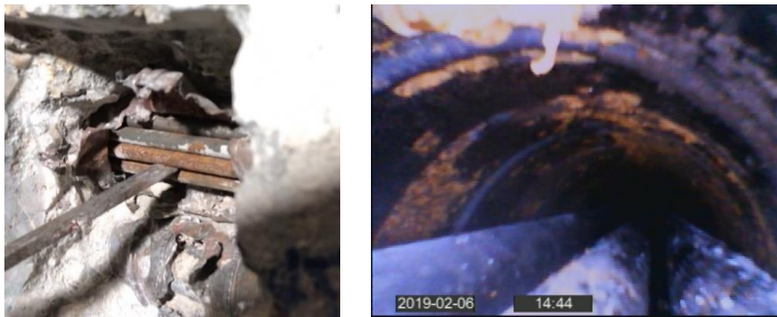
Fig. 20. Visual inspection of post-tensioning tendons in a rib (left), and endoscopy inspection inside a duct of the rib (right) (MASTRLAB 2019).
