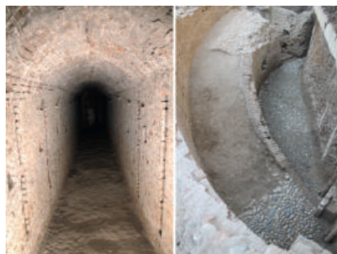
Fig. 3- Communication gallery between the ravelin and the citadel and access ramp to the rampart of the ravelin under excavation (photos by GEA S.A.R.T. s.a.s.)
