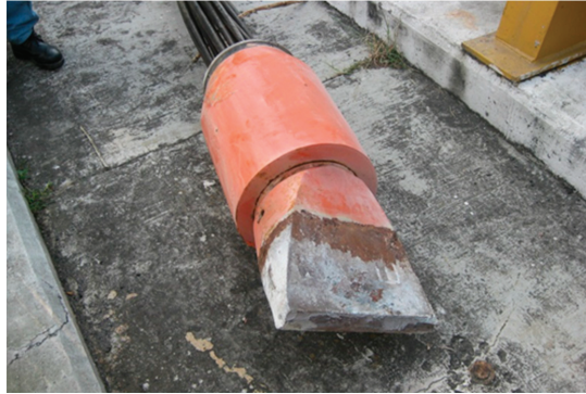
Figure 5. Failed anchoring element of cable 1 semi-harp 5 (T1S5).
