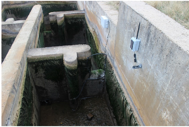
Fig. 2. Smart Fishways sensors implemented in a fish pass.
