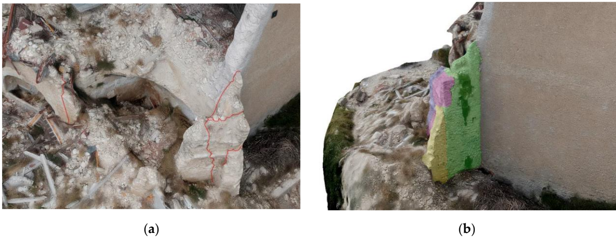
Figure 10. (a) Investigation of the anterior portion through the 3D mesh model textured by HD UAV images. (b) Recognition of the different portions of masonry not clamped or separated by cracks.
