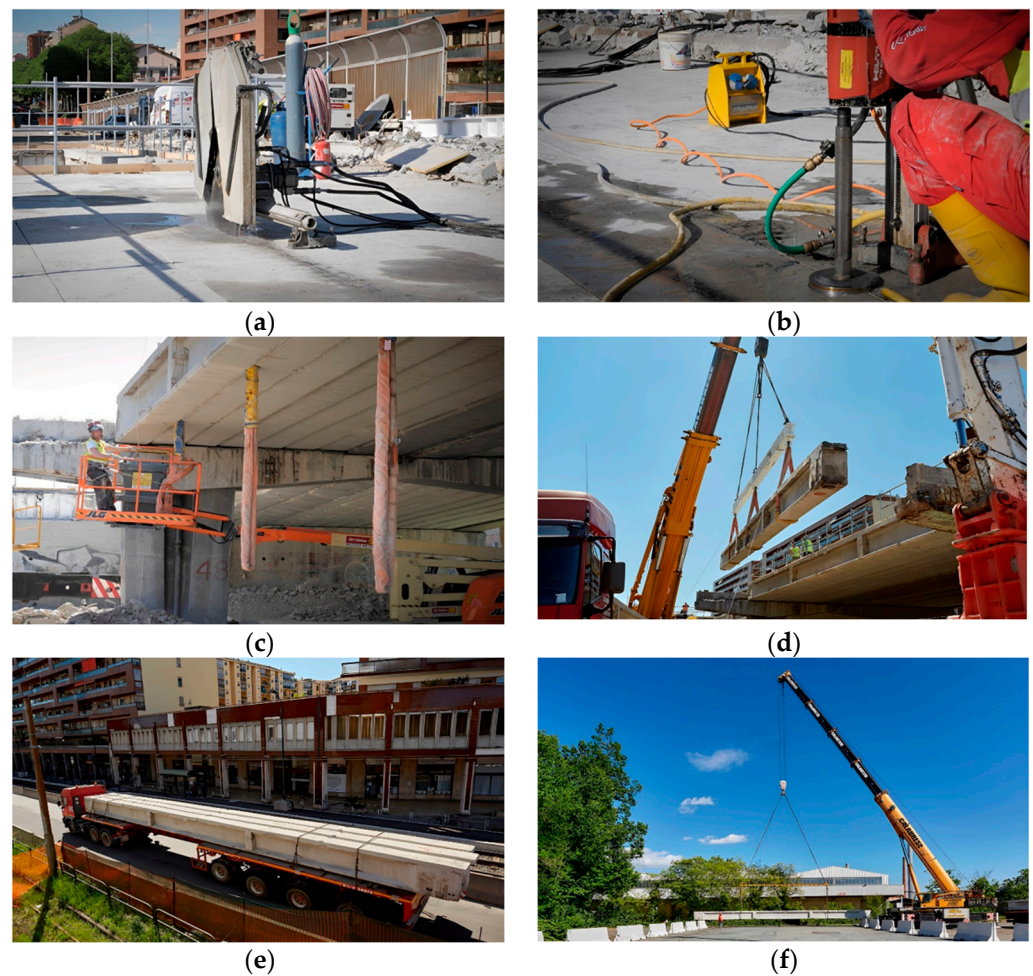
Figure 4. Deconstruction phases: (a) cutting; (b) drilling; (c) sling ropes; (d) lifting; (e) moving; (f) testing site setup.
