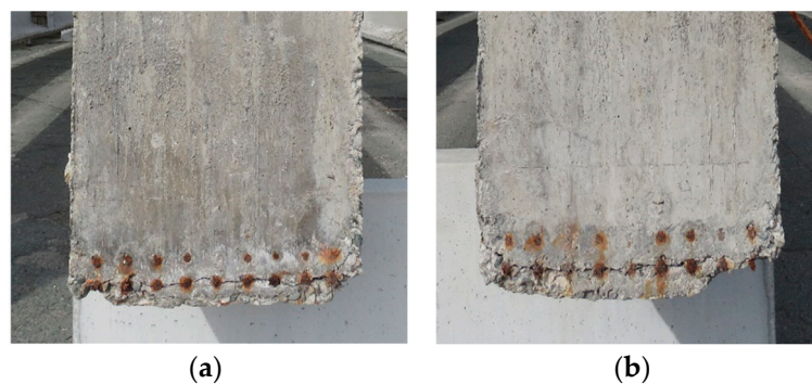
Figure 6. Cracks on the end of the (a) B3-P47/46 and (b) B4-P47/46 beams.
