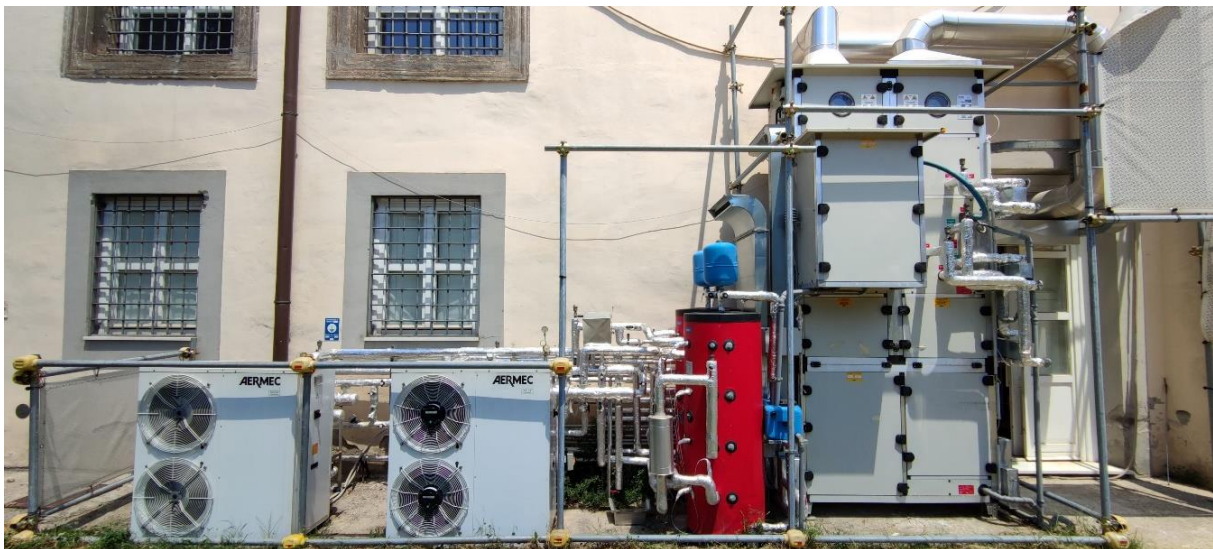
Figure 2. External view of the AHU of the SENS i-Lab.
