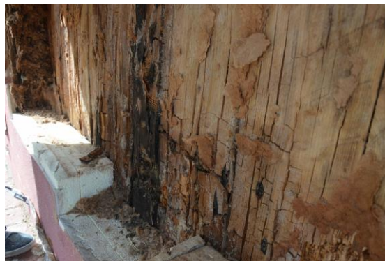
Figure 1 - Example of decay observed in a perimeter wall of a CLT building after just 2 years from construction
