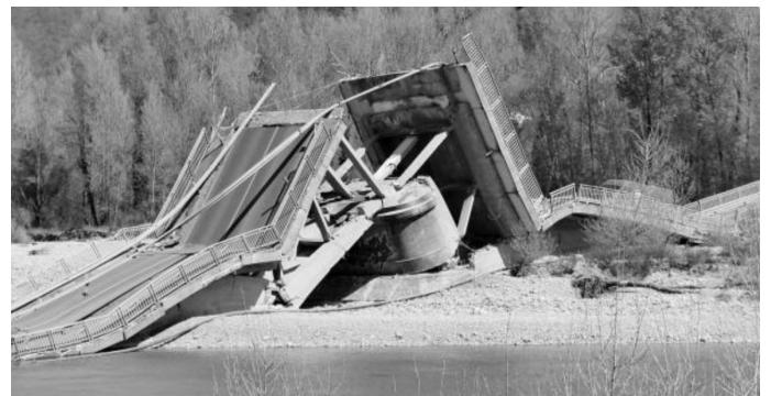
Figure 5. View of one of the piles of the bridge after the collapse.
