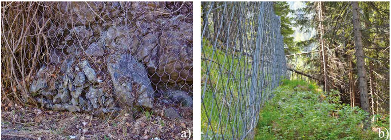
Fig. 2 – Accumulation of debris, due also to impacts with energy smaller than the design one (a), and impacts of element differing from rock blocks, i.e. trees after some severe or unexpected climatic events (b).
