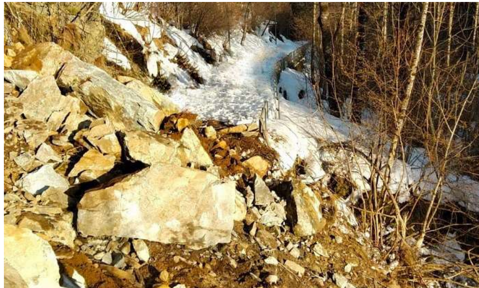
Figure 2. Rockfall event of 21 February 2021 (modified from: https://www.valsesianotizie.it/2021/02/21/leggi-notizia/argomenti/cronaca-9/articolo/rassa-frana-sulla-strada-per-piana-e-rassetta.html ; accessed on 24 July 2022).
