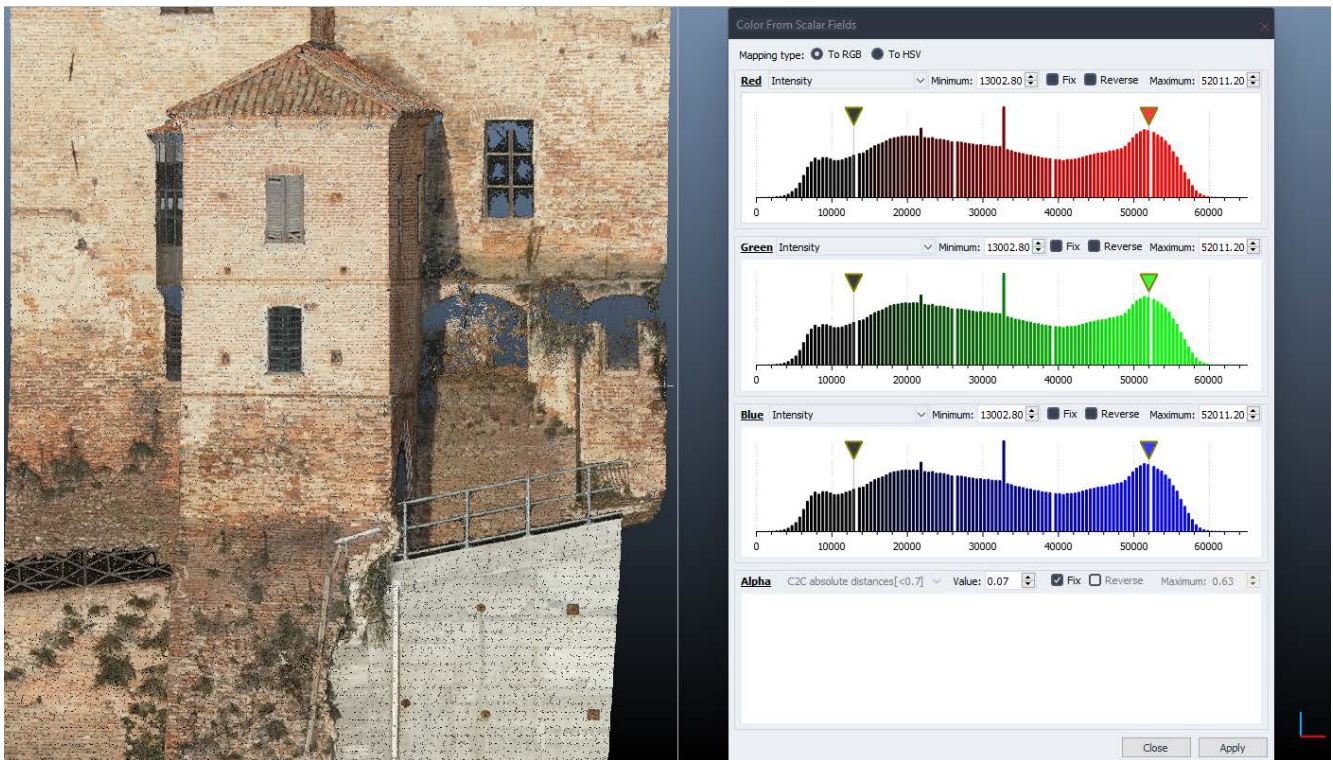
Figure 30. Radiometric values and red, green, and blue spectra related to the photogrammetric point clouds of the entrance tower.
