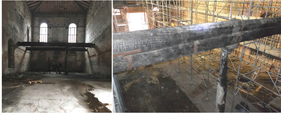
Fig. 5 Interior view of the Sala d'Armi “E” (left), detail of the burned wooden beam with wooden column (right). (Photo D. Ferrante, 2019)
