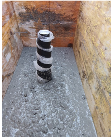
Fig. 3. Detail of the guided waves insulation during the casting in the framework of the concrete beam.
