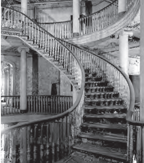
The Octagon, view of the helical staircase, in a state of neglect, 1970 ( https://www.theruin.org/blog/2016 ).
