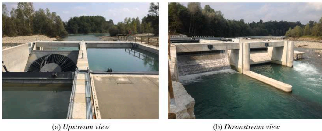
Fig. 3. VLHT installation in a canal, Mazzè, Italy. 2.60 m head, two VLHTs for a total of 54.2 m 3 /s, 5 m diameter each, 1000 kW of installed capacity and 25 m long derivation canal. Photo Courtesy Geasiste.
