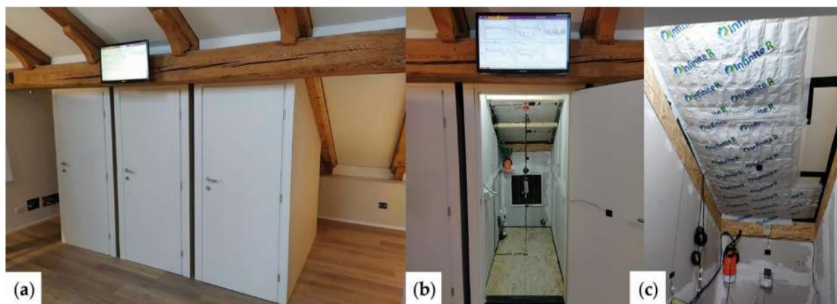
Figure 2. (a) The TRIS apparatus; (b) View of the internal space of a cell; (c) Installation of the Infinite R™ panels.
