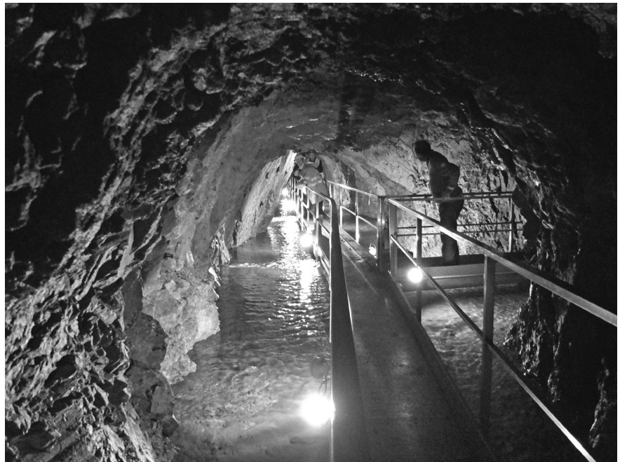
Fig. 8 – Hydrogeological monitoring of Tenda tunnel.
