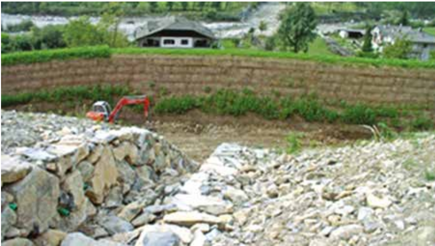
Fig. 1 – Example of a huge earth reinforced embankment, extended parallel the mountainside, for road and houses rockfall protection. Viewpoint is downward: in the uphill wall geogrids and lateral wire mesh adopted for the construction are still visible. Additional protective works against surface runoff have been done by means of local rock fragments and wood element for environmental sustainability (credits, structural testing and approval by C.Oggeri, Northern Italy).
