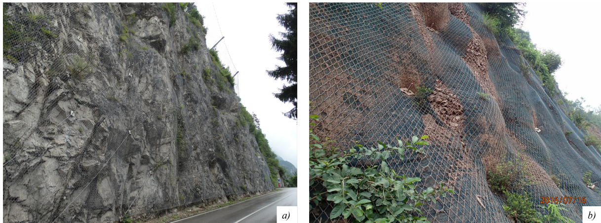
Figure 1. Reinforced drapery meshes with (a) retaining ropes, i.e., secured drapery, and with (b) spike plates, i.e., pinned drapery.
