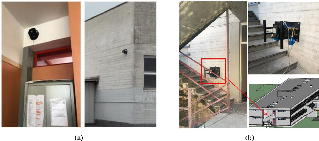
Fig. 4 – Installation examples of MEMS accelerometers (a) and vibrodyne positioning on the shear wall (b)
