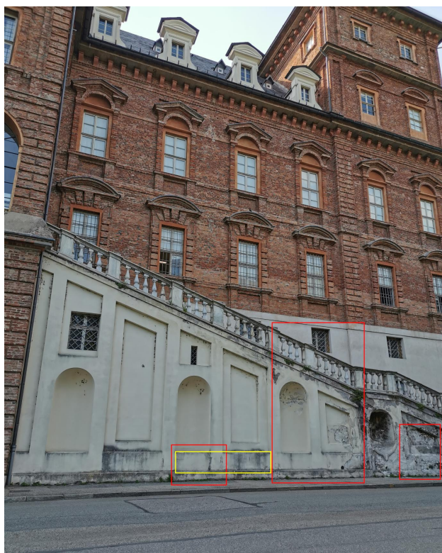
Figure 2. Castello del Valentino riverside (east) façade. The preliminary surveys are indicated with red and the detailed surveys with yellow color.
