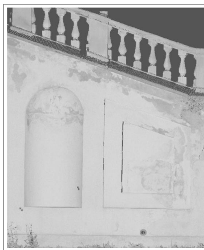
Figure 4: View of point-cloud pseudocolored with architectural surfaces' weathering indices (lower riverside façade)
