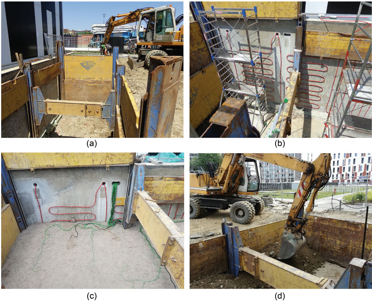
Fig. 4 Installation phases of the GeothermSkin system prototype on an existing structure: a excavation, b pipe deployment, c monitoring sensors deployment and d backfilling
