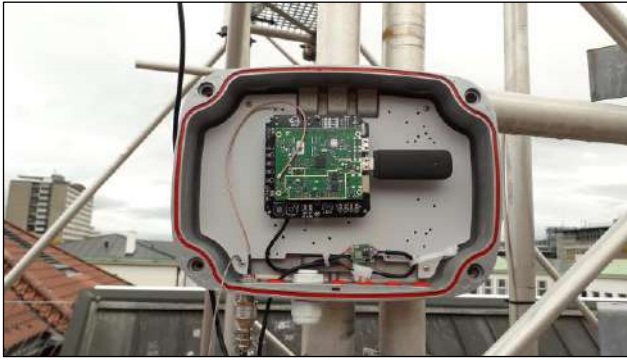
Fig. 3: LoRaWAN-Gateway at rooftop of HFT building 3
