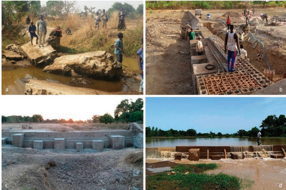
Figure 5. The rebuilding process in Toumbouba: (a) the old barrage down; (b) the building phase; (c) the wall complete; (d) the barrage working phase (Source: Authors’).
