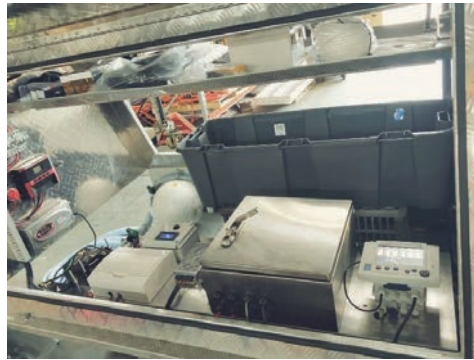
Figure 2. Interior spacing of the trailer, showing the wet area, communications box and sensor equipment.
