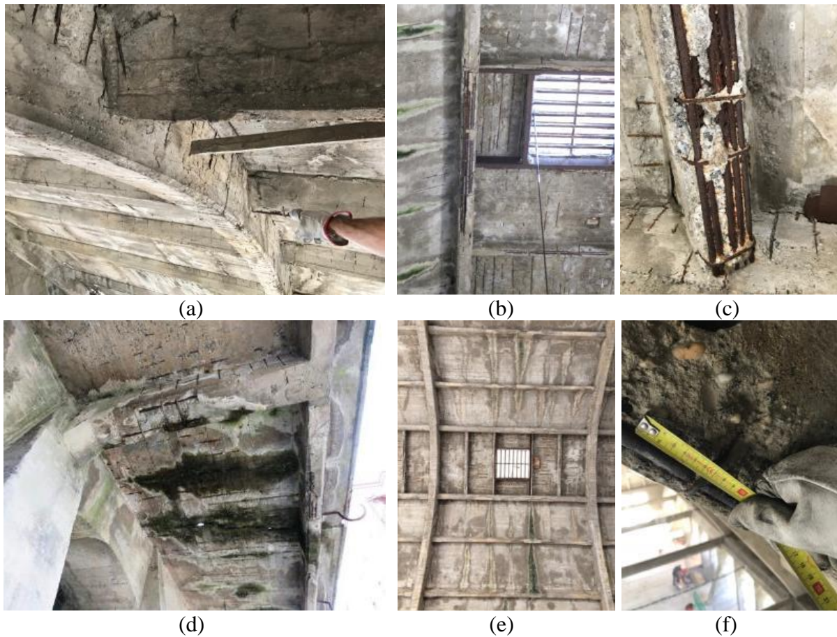
Figure 7: Damage and degradation on the building: (a) exposed rebars on the AR; (b-c) exposed rebars and detachments of concrete of the joists and roofing panels; (d) water staining and bio growth on the elements of the outdoors shelter; (e) a general view of the interior of the Paraboloid showing water staining and bio growth on the roofing panels; (f) a detail of the exposed rebars of a parabolic arch.
