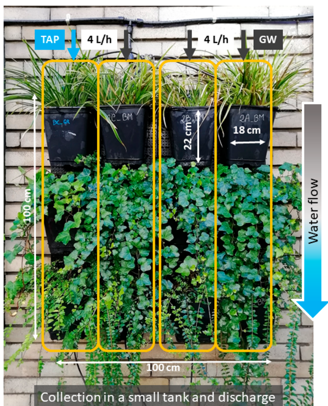
Figure 1. Modular panel of the green wall. All columns (marked in yellow) were identical except for the type of irrigation, and each worked independently. Three columns of this panel were fed with graywater (GW), and one was fed with tap water (TAP).
