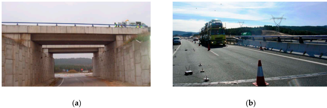
Figure 1. The skewed highway bridge: (a) Side view; (b) front view (during the measurements).
