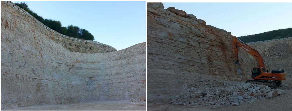
Figure 5. Quarry in limestone for aggregates, with two main joint sets; it is relevant the sub-horizontal system, with spacing of about 0.3–0.5 m. Left: blasting profile and few residual blast-holes in a vertical face 15 m high. Right: mechanical action of a hammer for detachment and scaling in a sub-vertical face 9 m high; scaling can represent an auxiliary procedure to solve mixed conditions (credits C. Oggeri and I. Cassone, quarry in South Italy).
