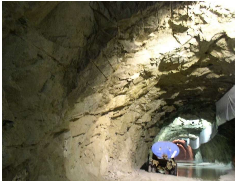
Figure 1. Contour of a tunnel wall excavated in a fractured granitic rock formation: both irregular joint surfaces and crack together with residual boreholes can be observed in close distance, proving the different results of round and damages for the same rock mass.(credits C.Oggeri, tunnel in western Alpine range, Northern Italy).
