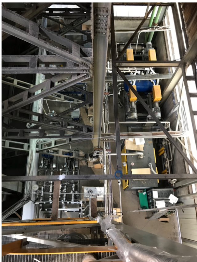
Fig. 9 Aerial view of the prototype Aria plant located in the Laveria building of the Carbosulcis mine, Nuraxi-Figus site. From bottom left, clockwise, the liquid pumps, the cryocoolers and the gas compressor.
