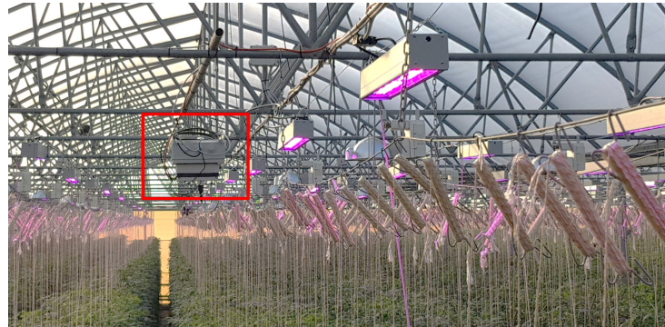
Figure 5. Sensors installed inside the greenhouse with the electrical cabinet containing the data monitoring unit hanged to the greenhouse cover.
