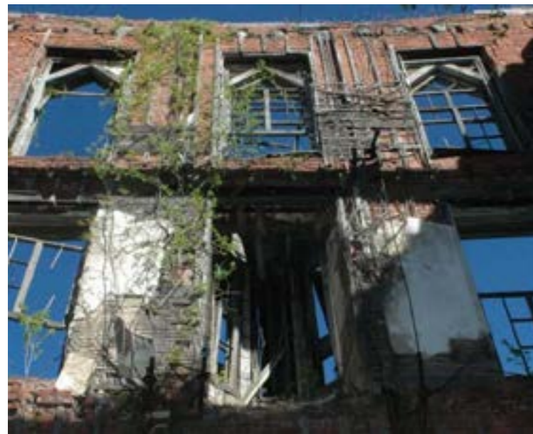
Detail from inside the masonry of the western façade (2009, John Milner Associates).
