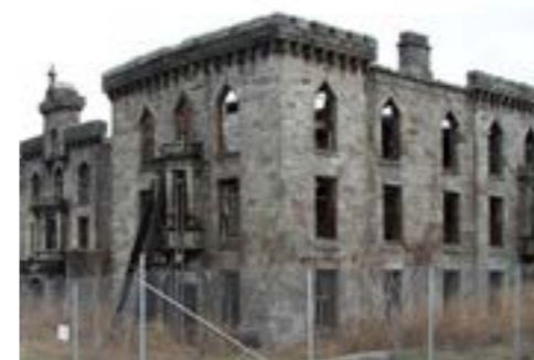
Smallpox Hospital, detail of the western façade after 1970 interventions, before 2009 consolidation works (www.theruin.org).
