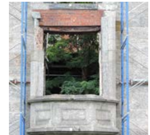
Caps and deficiencies, detail of the southern façade (2017, Balocco, Iurlaro, Lauri, Ravizza).
