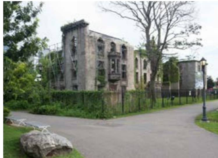
Smallpox Hospital, western façade, deterioration of the structure due to overgrowing vegetation.
