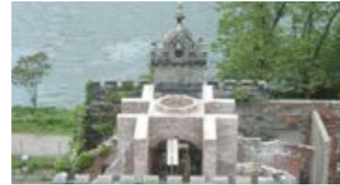
Details of the structure of the dome in the central wing before and after the reinforcement and reconstruction works (2009, John Milner Associates).
