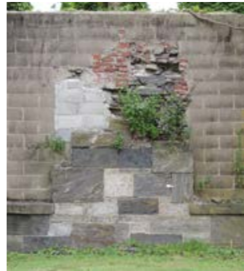
Western façade masonry, reconstructions project G. Cavaglieri (July 13 th , 2017, Balocco, Iurlaro, Lauri, Ravizza).
