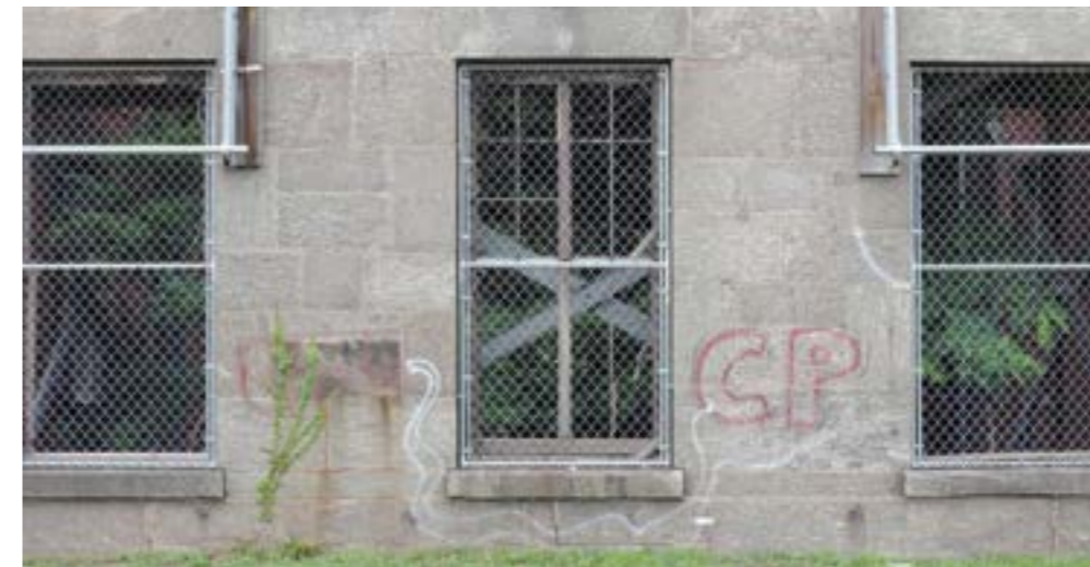
Anthropic degradation, detail of the eastern façade (2017, Balocco, Iurlaro, Lauri, Ravizza).
