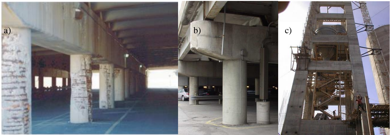
Figure 12 Highway bridge damaged by steel corrosion (a), Rehabilitated columns after twenty years of service (b), deficient industrial structure (c)
