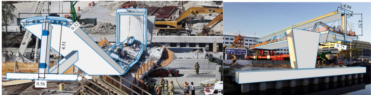
Figure 7 Image-based measurements of the collapsed Florida University pedestrian bridge for forensic analyses (reproduced from Peng et al., 2019).
