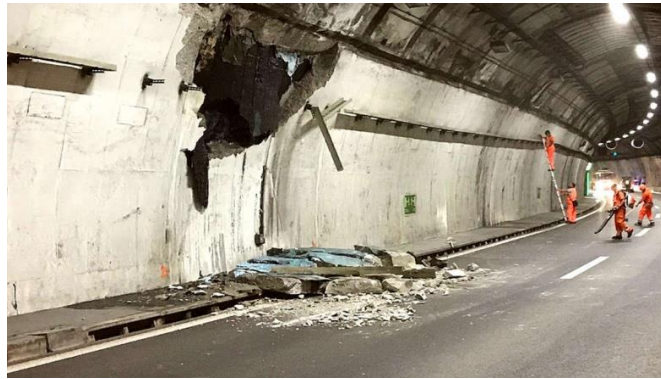
Figure 4. Local collapse of the San Salvatore Tunnel vault.
