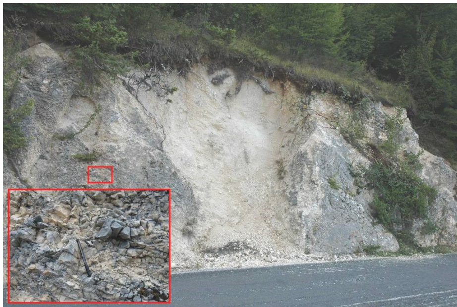
Figure 4.7. Failure in intensely fractured (i.e., sugar-cube) limestones (cataclasite).
