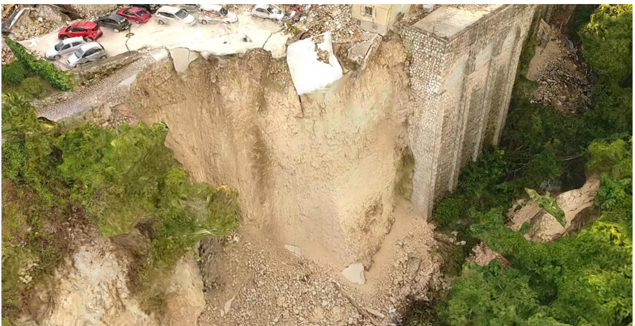
Figure 4.31. Model image of slope failure and possible retaining wall collapse (42.75109 N 13.27208 E).
