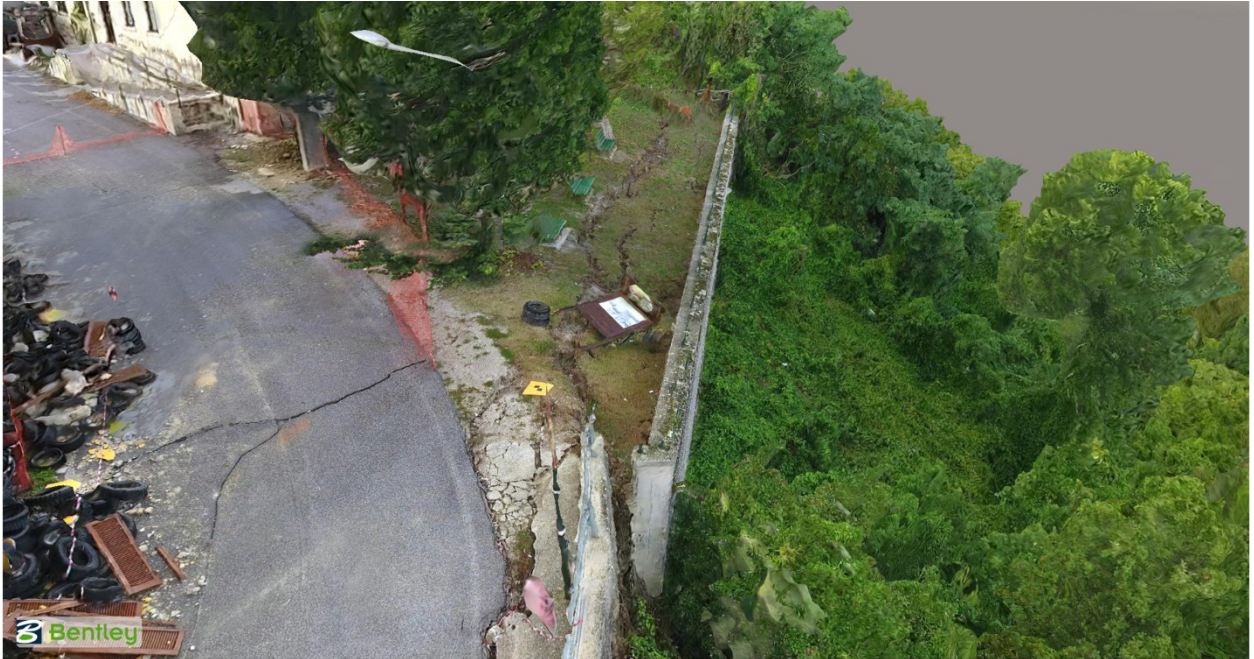
Figure 4.43. Rotated retaining wall and subsequent graben behind the wall. Soil settlement between 45-50 cm behind the wall, and formed cracks up to 45 cm in width (42.69446 N 13.24980 E).
