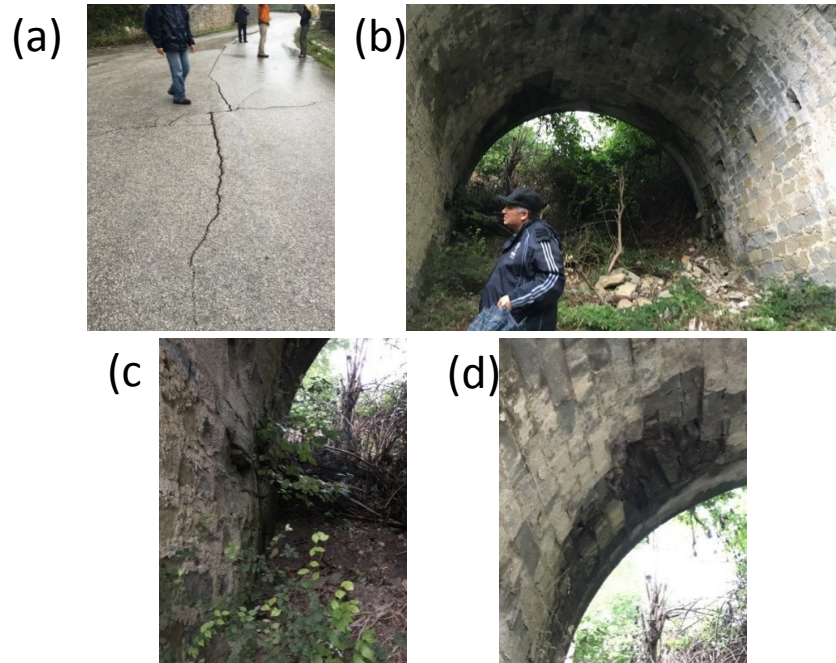
Figure 6.7. Masonry bridge along the Trisugo route (42.735981 deg, 13.254862 deg): damages on the road (a), overview of the bridge (b), abutment (c) and partial collapse of the interior part of the arch (d).
