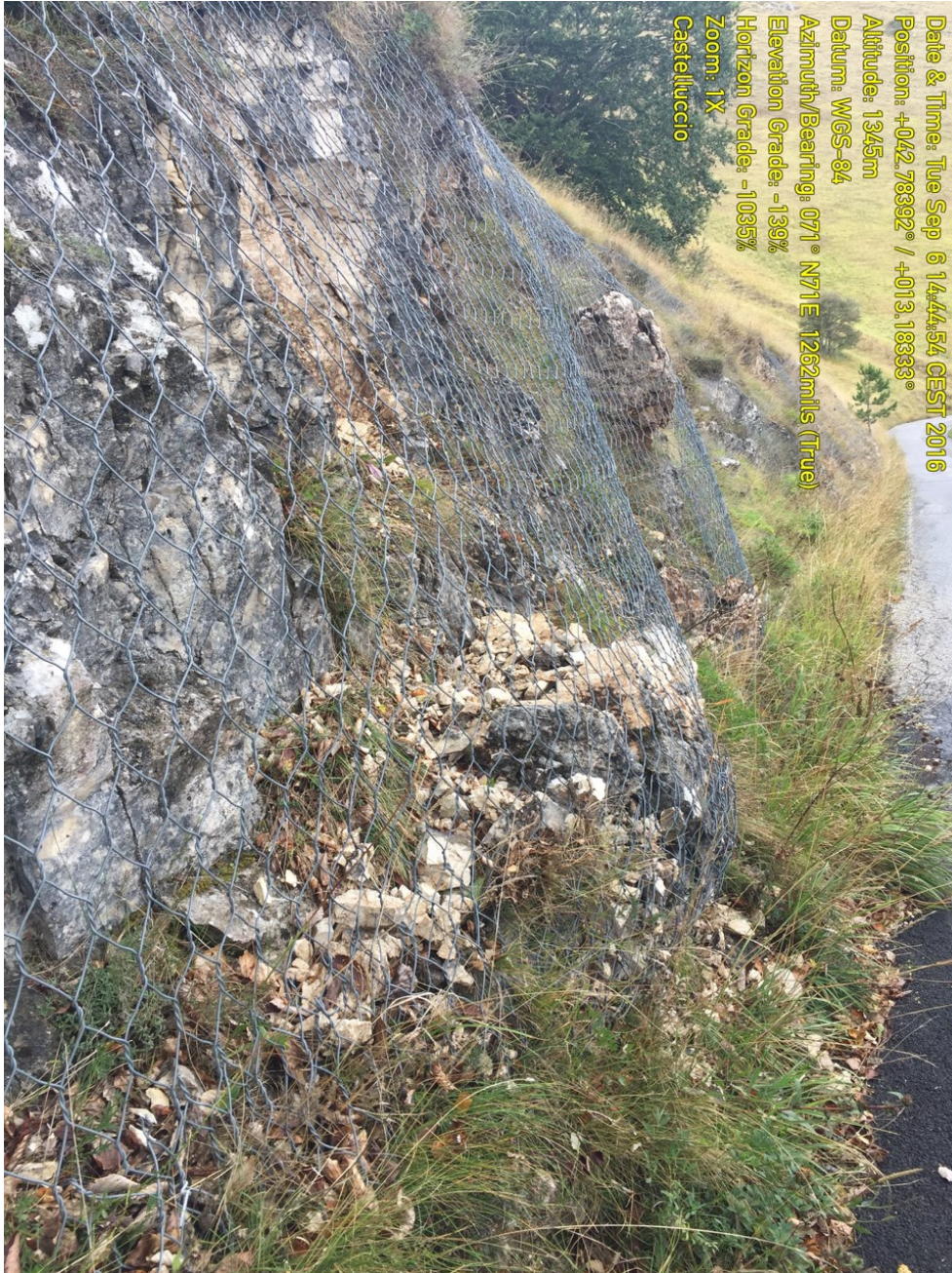
Figure 4.20. Rock-net protection with captured debris from the earthquake, including minor small debris in the foreground and a large ~0.5-m block in the background (42.78392 N 13.18333 E).
