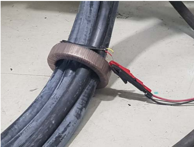
Fig. 5. Test specimen installed on the power converter cables.
