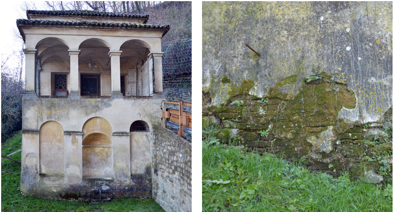
Fig. 2. Serralunga di Crea, Sacro Monte, Chapel 1. Main façade (right) and damage at the base of the northern façade (left).
