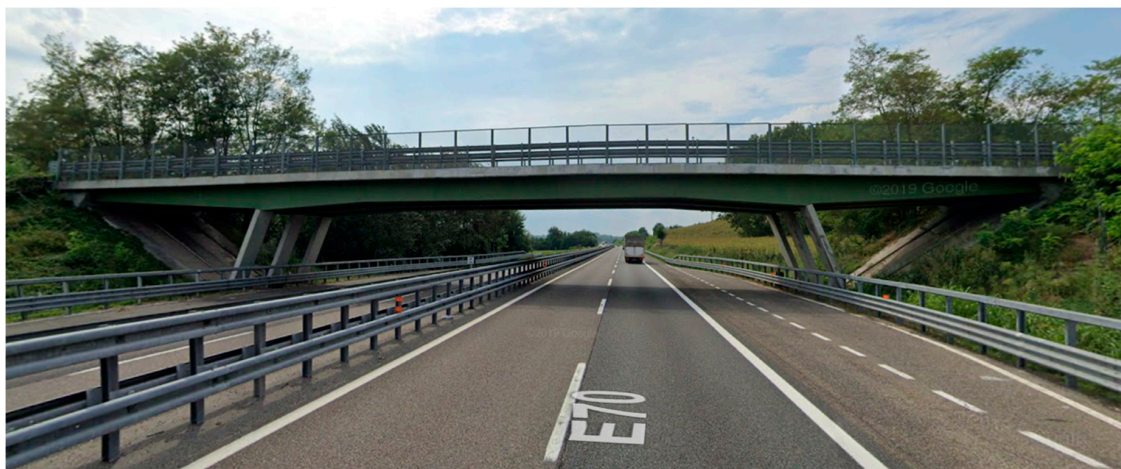
Figure 7. Street view of one of the overpasses of the Italian Highway A21 (source Google Maps).
